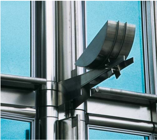
Detail view of baffled uplight
